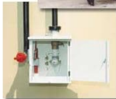
Ground Level Spill Box
